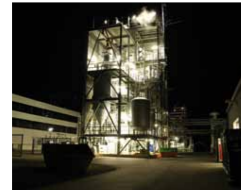
The pilot facility of the slagging bath gasifier at the Freiberg site is operated in close cooperation with the Institute of Energy Process Engineering and Chemical Engineering at the Technical University Bergakademie Freiberg. The facility is used for tests involving various solid carbon carriers, such as biomass and plastic-containing waste.
